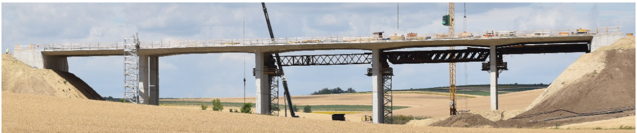
▲ Schematic arrangement of the expansion joint for integral bridges and the first application in the Satzengrabenbridge
